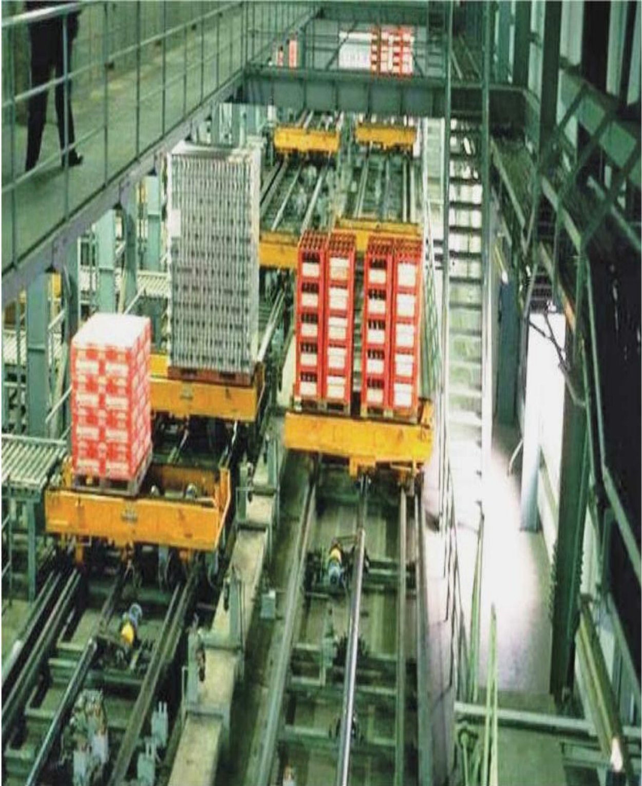
Figure 9.19 Pallet conveyors feeding vertical transport systems are a common means of interactivity movement in multistory warehouses.
