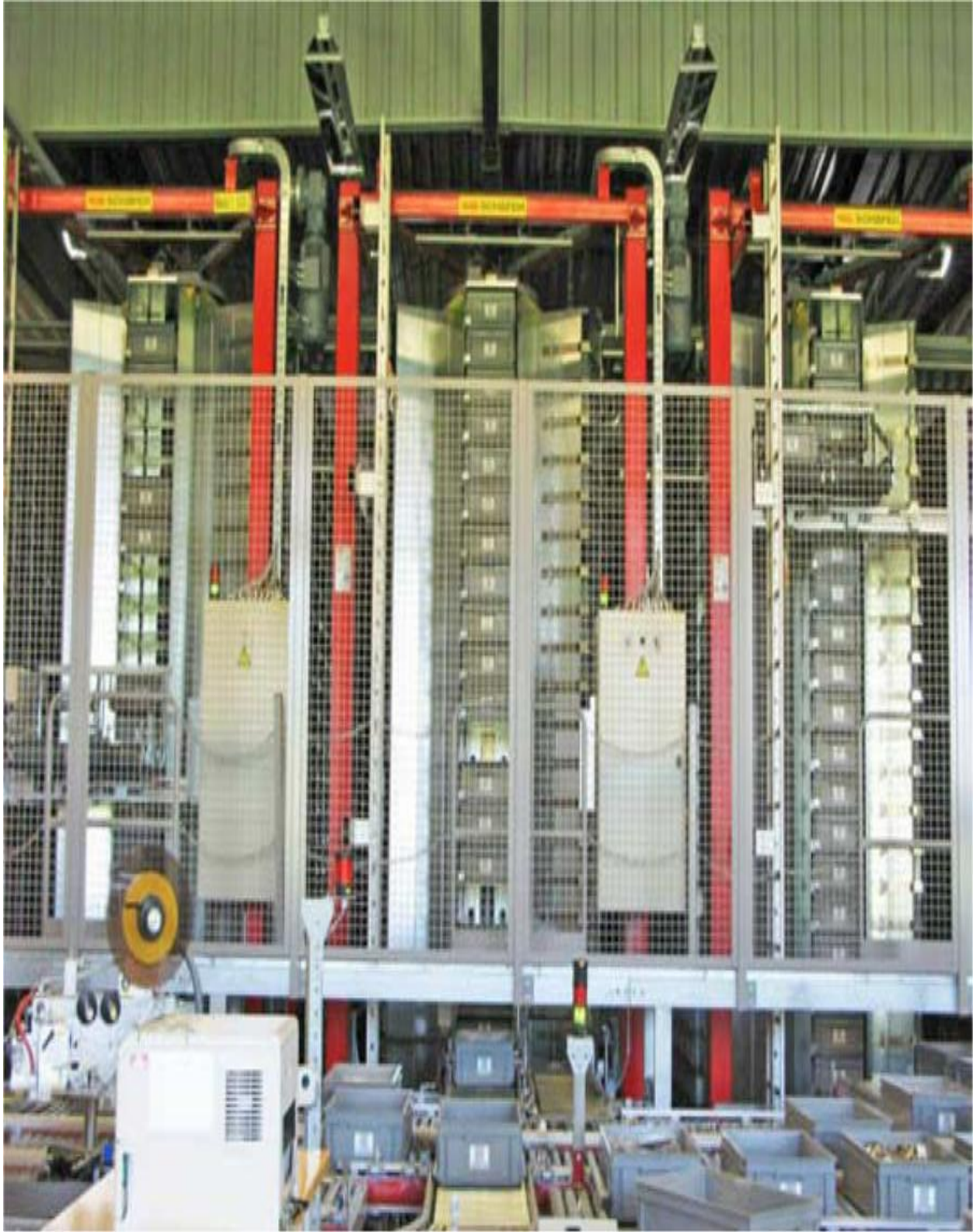
Figure 7.46 Horizontal carousel storage and retrieval system with
