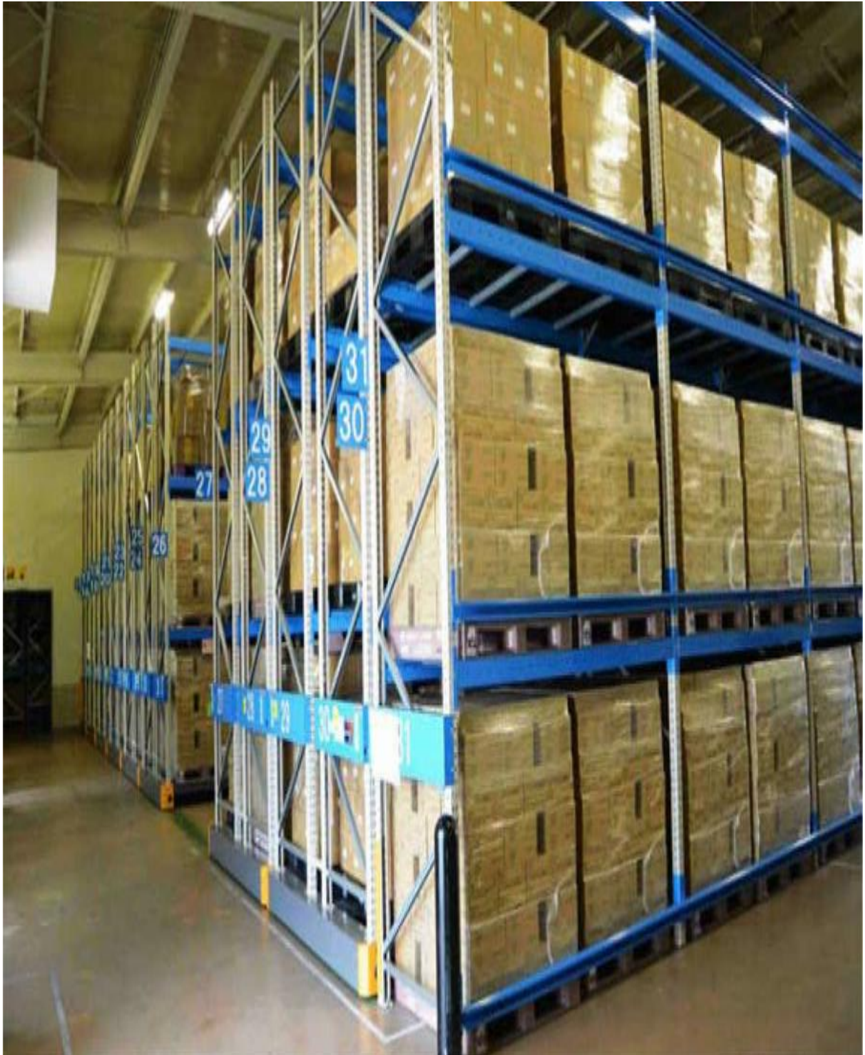
Figure 5.25 Mobile pallet rack installation.
