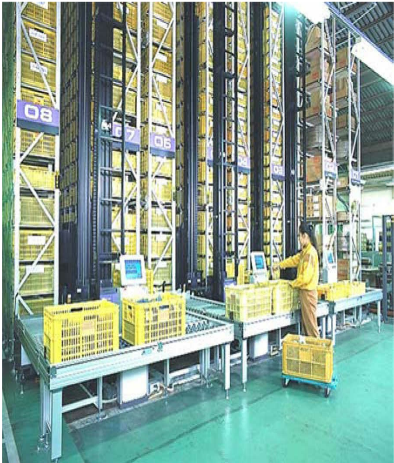
Figure 7.52 Even miniload systems can be configured with mobile aisles, as is the case in this installation.
